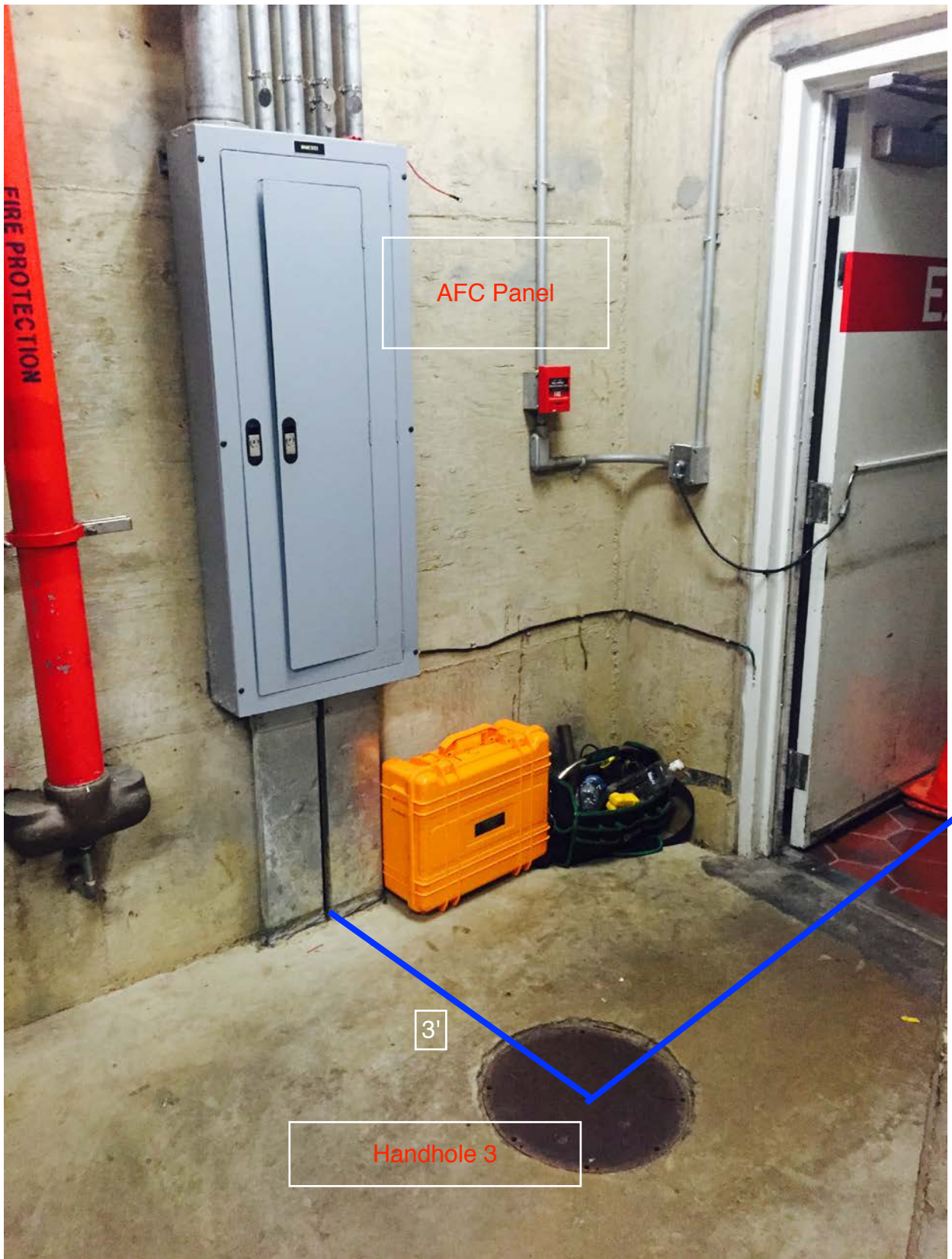
Photo #2: Existing duct run from Handhole 3 to AFC panel (Room 101)
